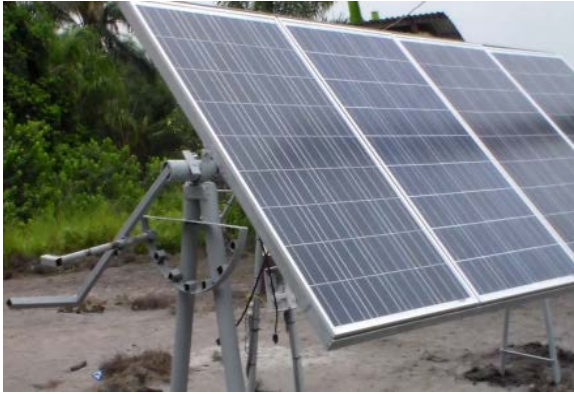
Figure 5c: A small-scale solar array structure of Configuration C with manual tilting system.
