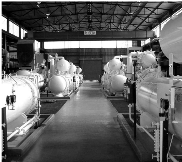
Figure 1: Chiller room at a large industrial plant
